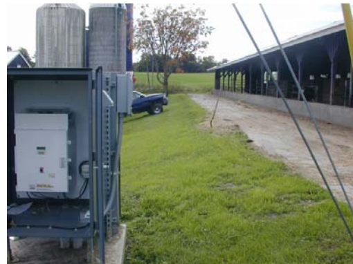
A weatherproof enclosure (opened for the photograph) houses inverter and cable leads from anemometer and wind vane
