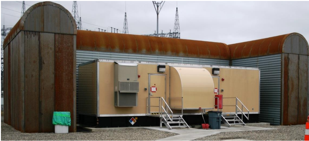
Security Diesel Generator
