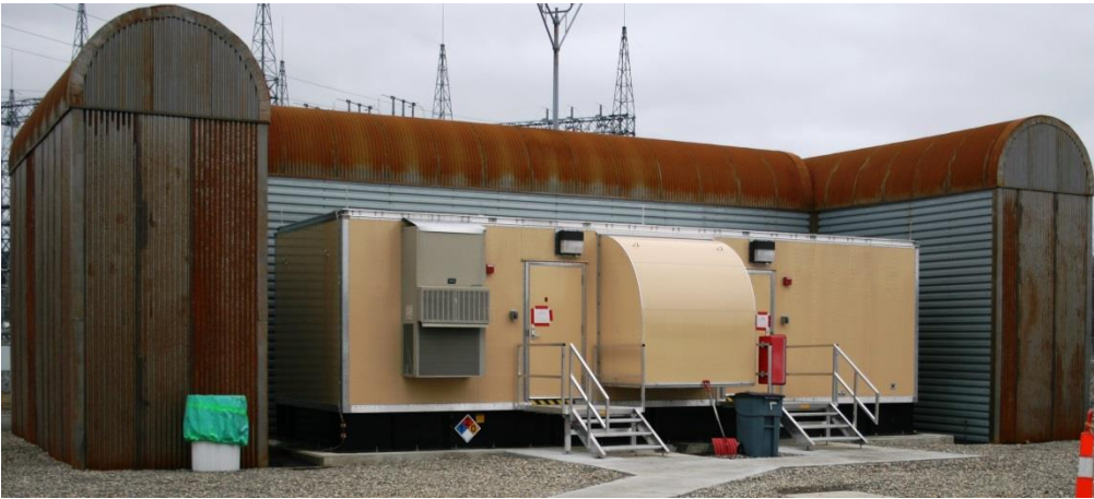
Security Diesel Generator
