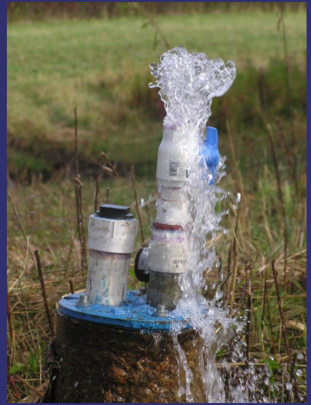
Overflowing well, Hinesburg
