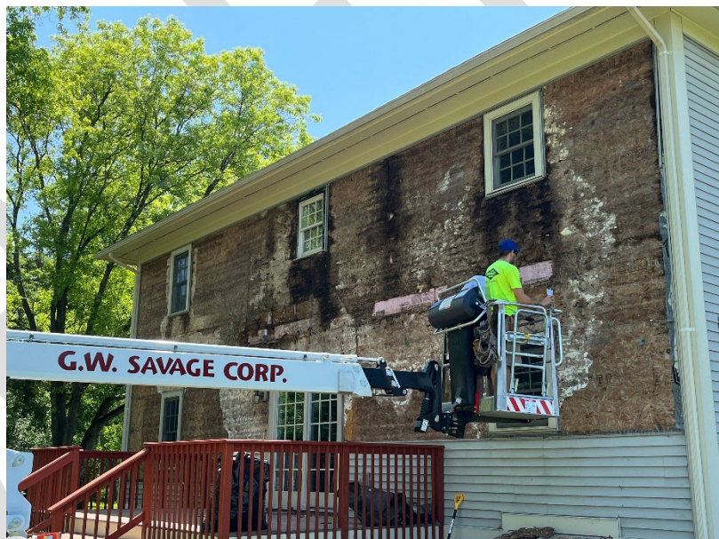
Figure 2. Remediation crew repairing relatively new Vermont home extensively damaged by moisture from indoor air that migrated into the walls (courtesy of Jim Bradley, Hayward Design Build).
