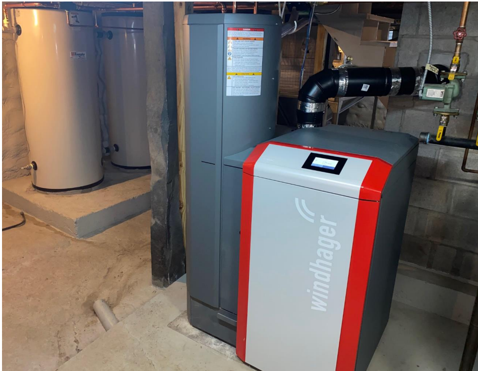
Figure 6 - a new pellet system installed in East Montpelier that replaced an old coal boiler.
