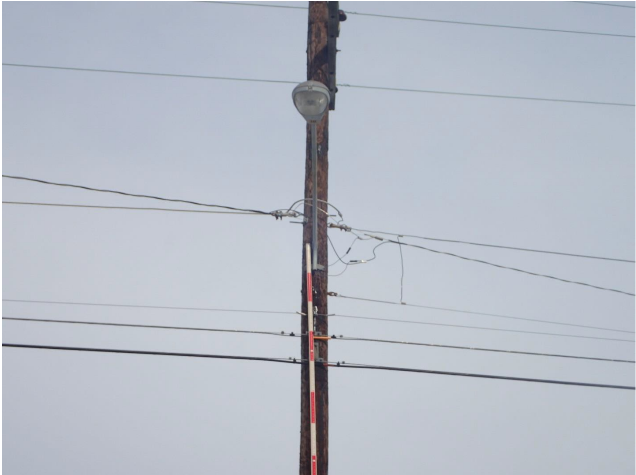
Figure 3 - Ungrounded Luminaire clearance to communication cables
